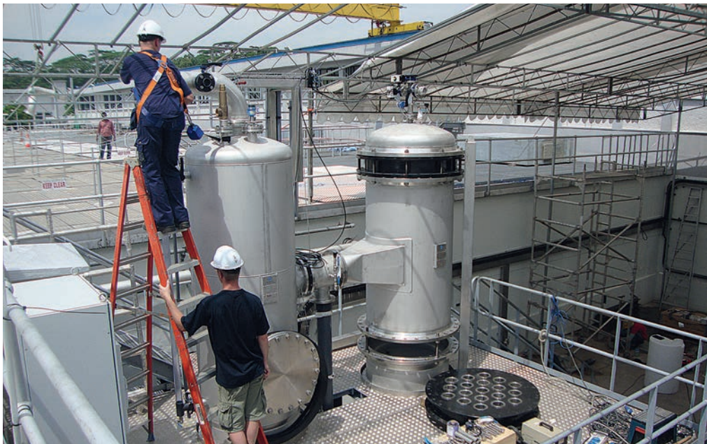
CeraMac-19 vessel (right) and backwash tank (left) being installed into an existing sand filter bed at Choa Chu Kang Waterworks, Singapore.
